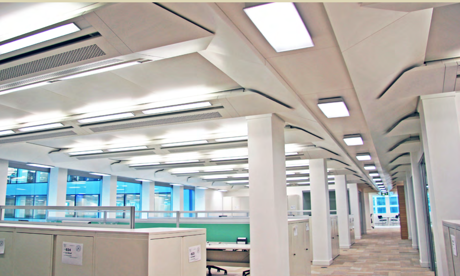
55 Baker Street original installation - 2007
