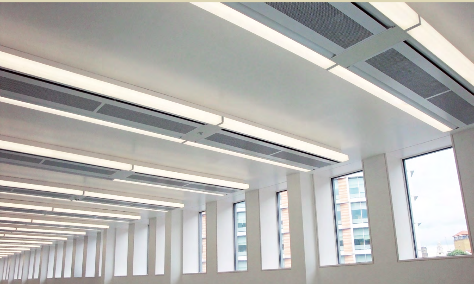
65 Southwark Street original installation - 2012
