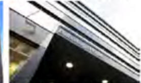
Bidborough House London, UK - 2008 Active Chilled Beams
