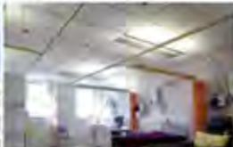
Royal Sussex Hospital Brighton, UK - 2002 Active Chilled Beams
