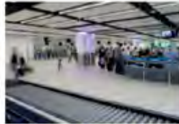
Gatwick Search Area London, UK - 2011 Passive Chilled Beams
