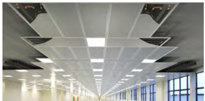
Exposed grid for lay-in “chilled tiles”
